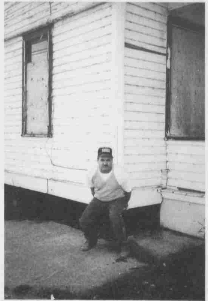
Terry from Wyser Contracting "lifts" an old house to new heights to house more people. A new foundation and other renovations will create 11 self-contained units with 1 bedroom, full bath and kitchen. Total project cost is around $200,000, including $99,000 from the RRAP program. Look for the re-opening of this historic house at 9315 108A Avenue on October 1. Photo by Kate Quinn
