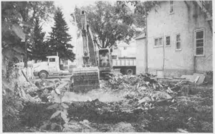
A bulldozer finishes the job on a derelict house on 92nd Street. This house was a source of problems for neighbours and the scene of a major fire in October, 1997. A new duplex is rising on the site of this old eyesore. Photo by Kate Quinn
