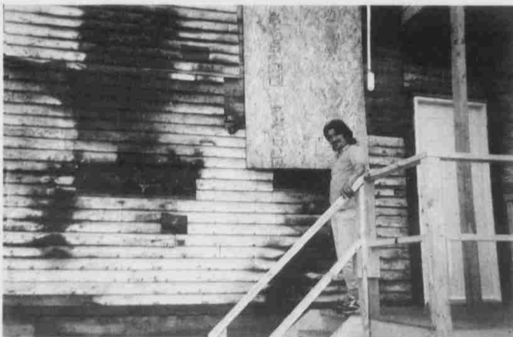
Kyle Laboucane stands on the back stairs of Vancouver Rooms. The rear of the building has boards covering blackened holes from the recent fire, and two suites still need to be repaired.
