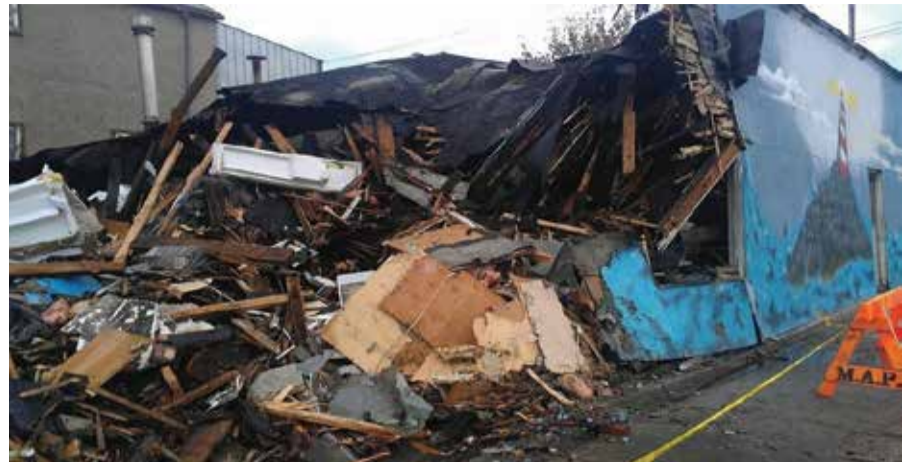
All that remained of House of Refuge after the fire. Clara Gladue
