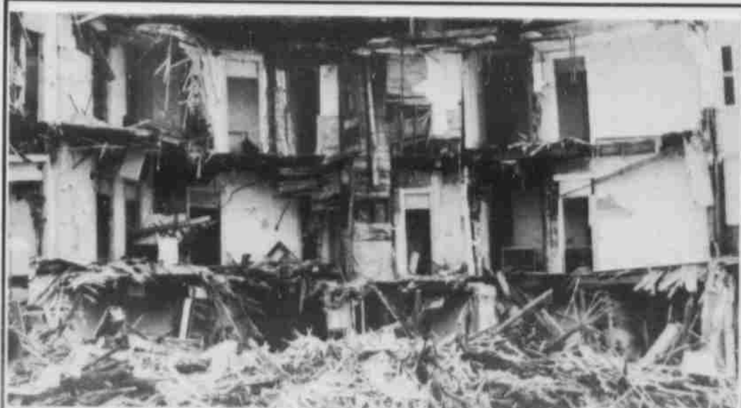
The old makes way for the new: Alex Taylor Apartments demolished for new condo development.
