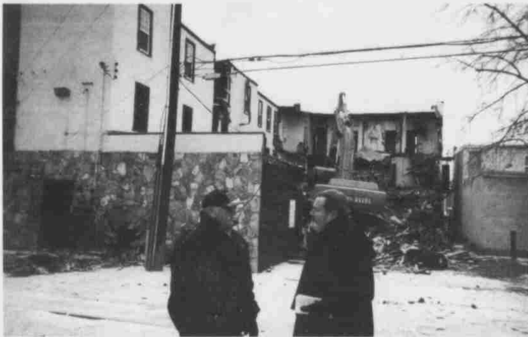
Member of Parliament, Peter Goldring (right), came to watch the demolition of the International Hotel, 96 Street & 103A Avenue.
