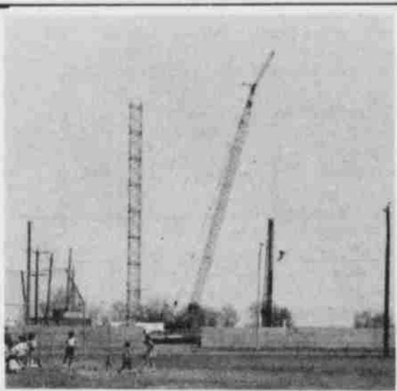
Highland Court, once a refuge for tenants on low income, is in the process of being replaced by a highrise complex.
