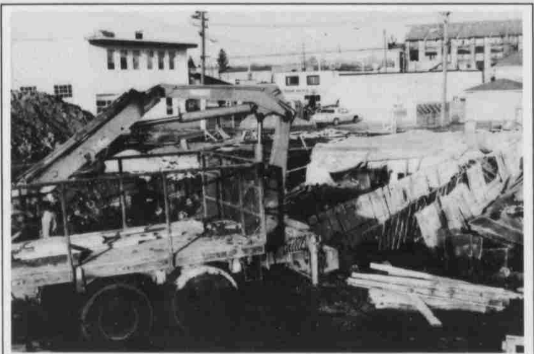
Operation Friendship Housing Society is constructing a twenty unit self contained apartment building at 95th street and 110 A Avenue. It is scheduled for completion at the end of July, 1992. The target population is seniors who qualify for subsidized rents and have had difficulty finding secure housing in the community.
