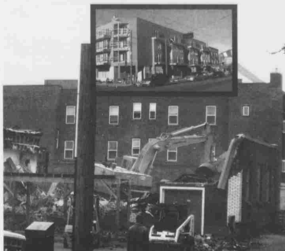
CHANGING STREETScape | Demolition of the Brew for Less store at 108 Avenue and 95 Street makes way for the second building planned by developers Tony and Peter Pino. The first building (inset) with its 36 residential units and main floor commercial space is substantially complete. The second building, which will be a twin of the first, is expected to be constructed within a year.
