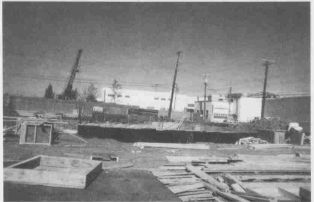
Construction on the new Urban Manor is well underway. Susan Irvine, who works at Urban Manor, said they are hoping to move in by May or June, 2002. The new building will be three stories high, and designed for the hard to house and those with mobility problems. There will still be some four man dorms, but the beds will be separated by pony walls for more privacy. Photo by Linda Dumont
