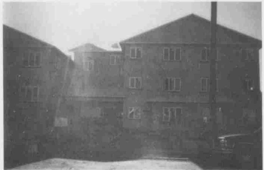
Construction is well under way for the Rotary Millennium House, a 25-unit single dwelling residence located on 106 Avenue west of 96 Street. The City Centre Church Corporation and the Downtown Rotary club are major partners.
