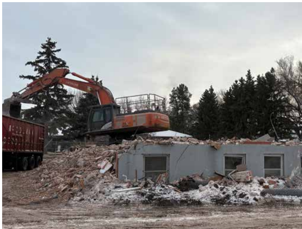
Demolition work at the site of Atonement Home in late December. Paula E. Kirman
