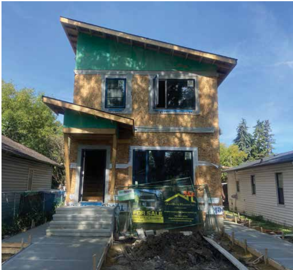
A property in McCauley that was redeveloped after being cleaned up by the PPI. Supplied by the City of Edmonton
