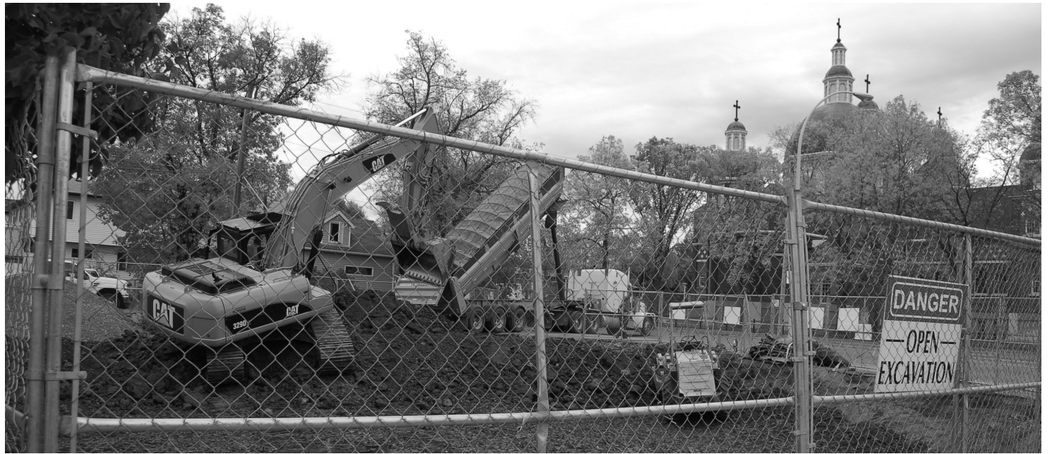
Work being done at the site of the former Husky station on 108 Avenue and 97 Street. Paula E. Kirman
